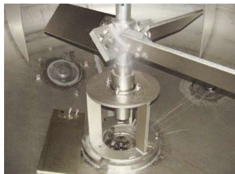
Detached agitator blade in mixing vessel due to broken bolts
