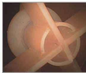
■ Crack in Attemperator
